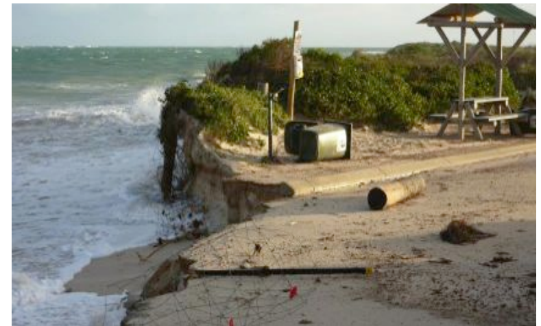
Figure 5: Coastal recession at Thirsty Point – photo Paul Robb.
