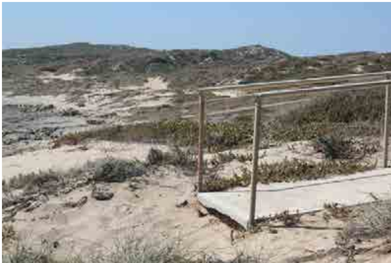
Plate 17: Erosion under access ramp
