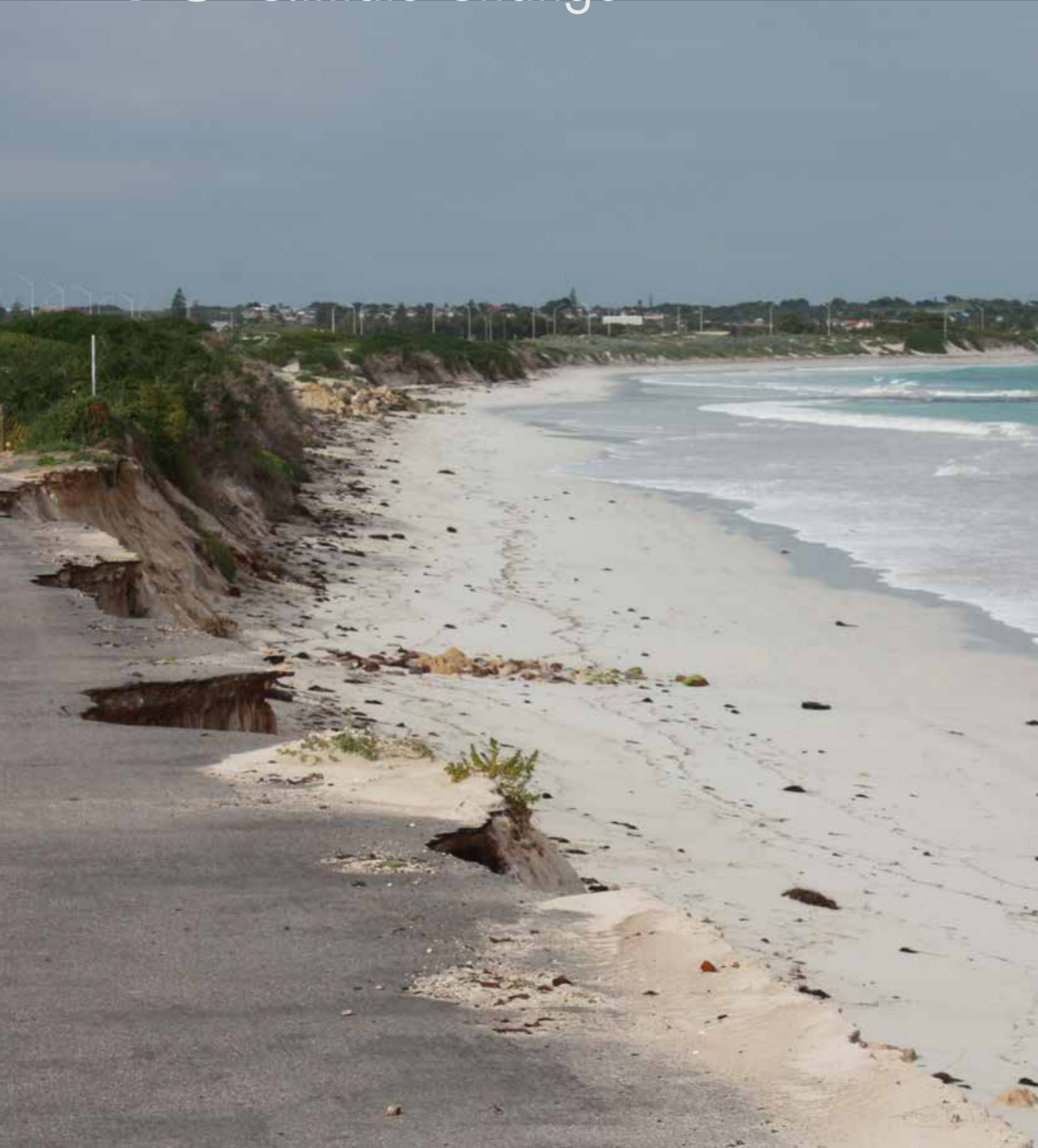
^ Erosion Greys Beach, Geraldton.
