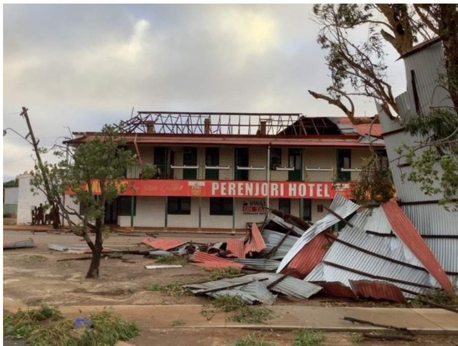
Figure 3: Serious infrastructure damage to the Perenjori Hotel after Seroja. Image courtesy of Kirk and Silvia Pohl
